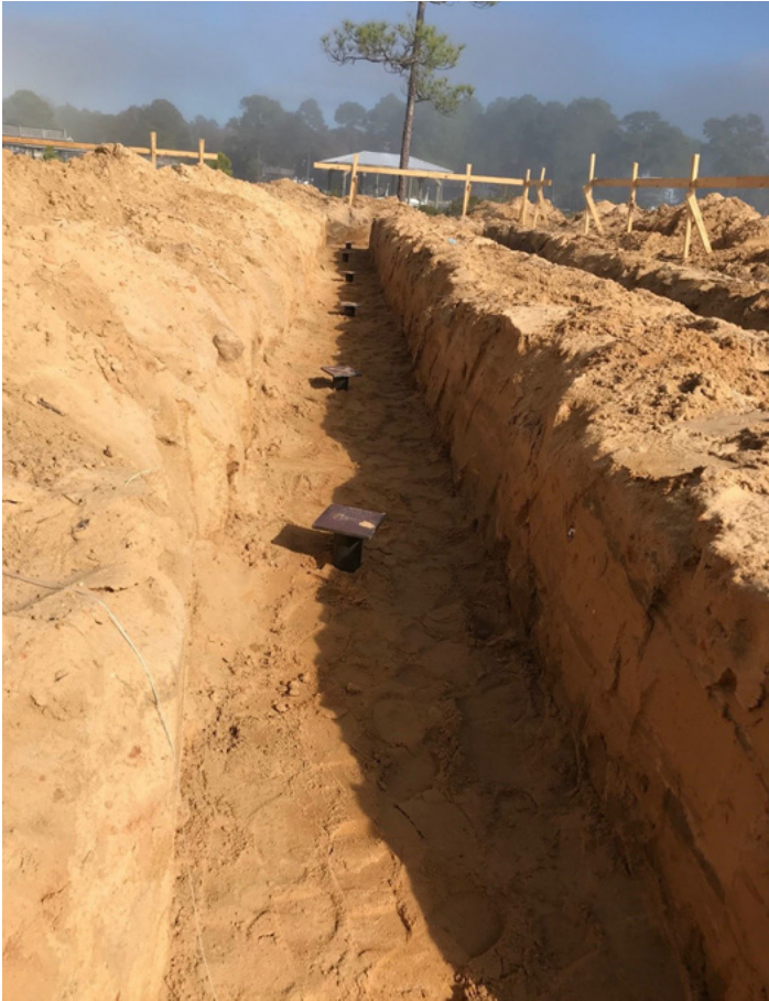
Completed pile system with new construction cap to allow for connection to the concrete grade beams.
